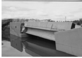
M-57 over Northwood Creek. Cause – Road improvements increased pressure flow.
