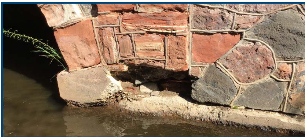
Deterioration of the south wall of the Silver River culvert (Courtesy of MDOT)
